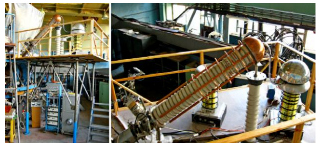
Fig. 4. General view of HIBP system at Uragan-2M torsatron with beam control and data acquisition system (left). Upper platform with primary beam injector, power supply +200 kV, emitter heating and extractor power supplies system, grounding system (right)
