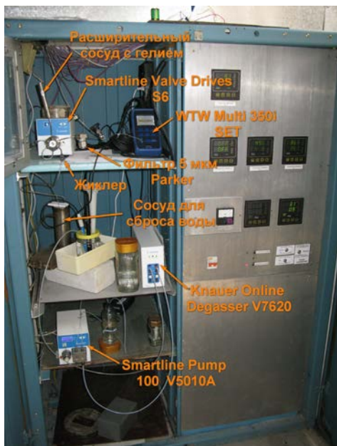
Fig. 2. General view of the control rack
