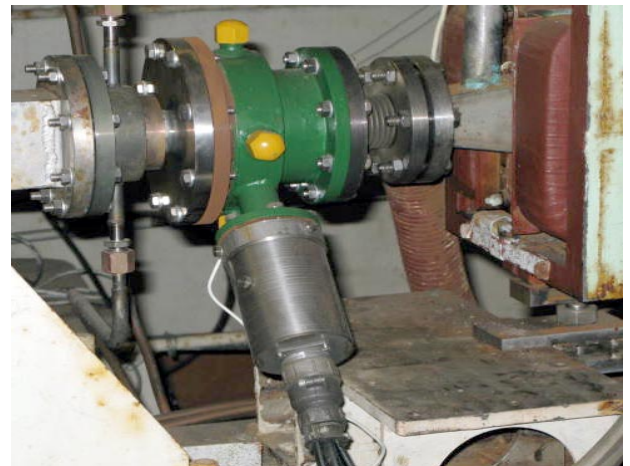
Fig. 5. Appearance of the protective collimator unit (on the left) and transit sensor (in the centre) at the exit of the accelerator LU-10
