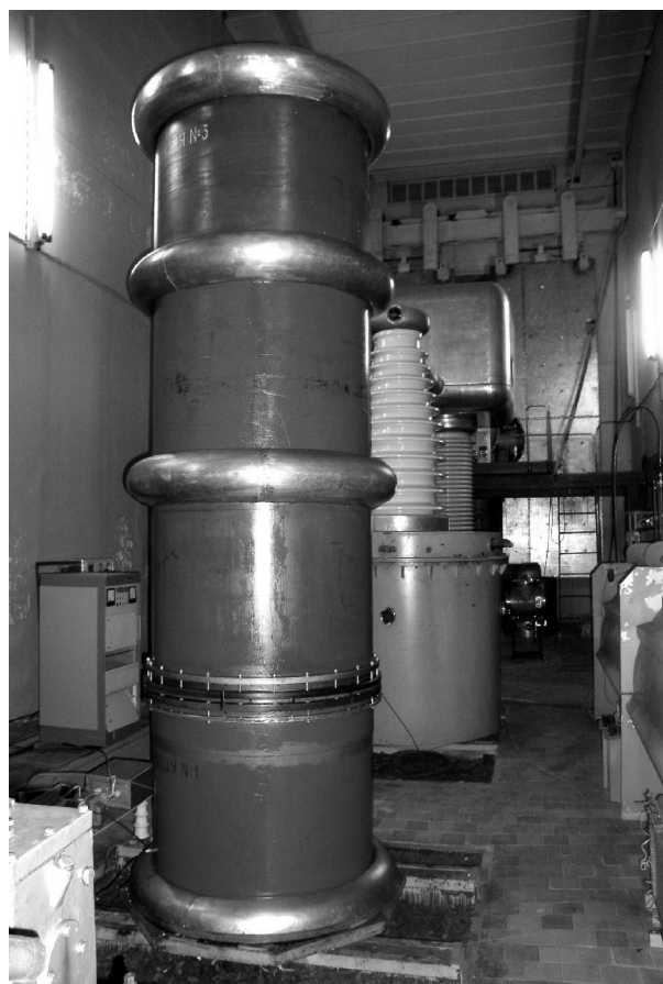
Fig.1. The equipment inside the injector high-voltage room: DSR, pulse transformer and high-voltage shield of IS power supply
