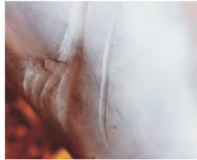
Fig. 2. Example of dents on pipe.
