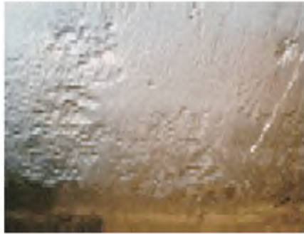
Fig. 1. Example of corrosion defect on pipe.
