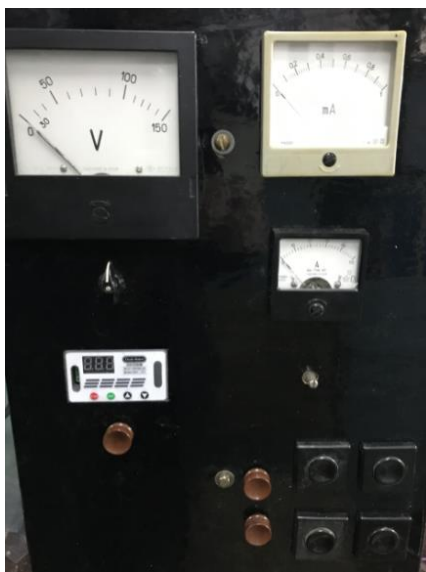
Fig. 2. Control panel of EPP device
