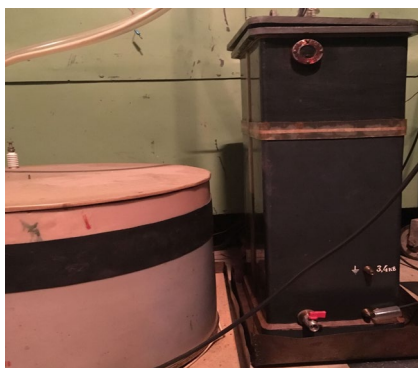
Fig. 6. Modulator output transformer and high voltage stabilizer
