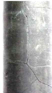
Fig. 7 Cracks in the CCFBPyC, ShP-13
