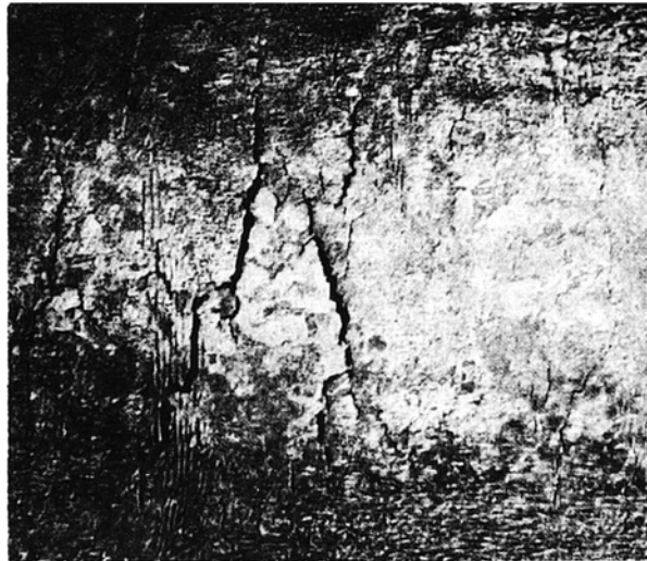
Fig. 2. External appearance of deep cracks on the outer surface of the steam line pipe.
