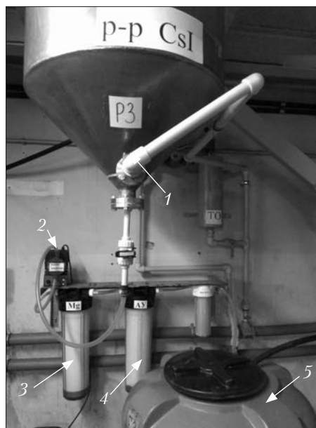
Fig. 2. The view of the experimental-industrial node of CsI purification by filtration through cartridge filters filled with magnesium and carbon: 1 – heat-exchange apparatus (titanium); 2 – metering pump; 3 – Mg-filled cartridge filter; 4 – activated carbon-filled cartridge filter; 5 – capacity for the filtered solution
