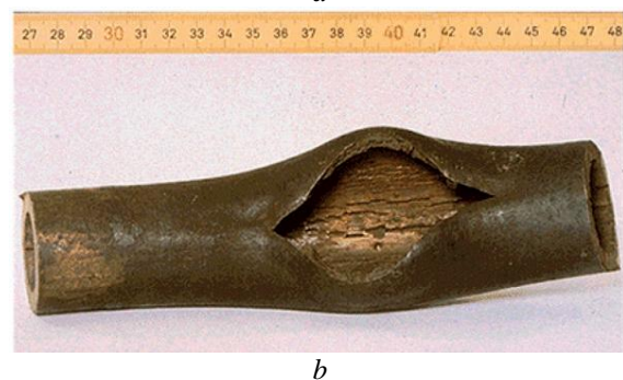
Fig. 2. Fragment of a crack in the metal pipe [43] (a), high temperature hydrogen attack of carbon steel cooler pipe of a heat exchanger [32] (b)
