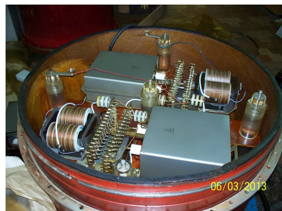
Fig.5. General view of two installed MD cascades with the new chokes
