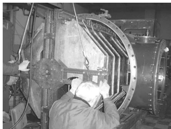
Fig.10. Mounting of the resonator in a vacuum tank
